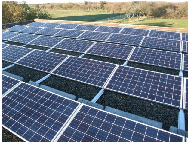
Statkraft's first solar park in Germany was constructed in 2018, next to the hydropower plant in Dörverden. The 750 kW park is a test site for the combination of solar power and batteries.
